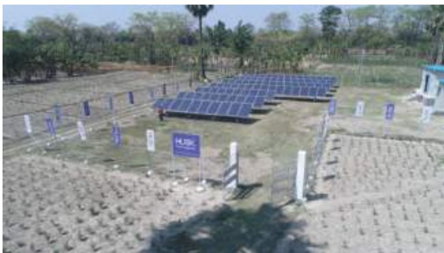
Figure 6.5: HUSK Solar Plant
