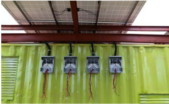
Four PV string combiner boxes in Kanyegaramire mini-grid during construction
