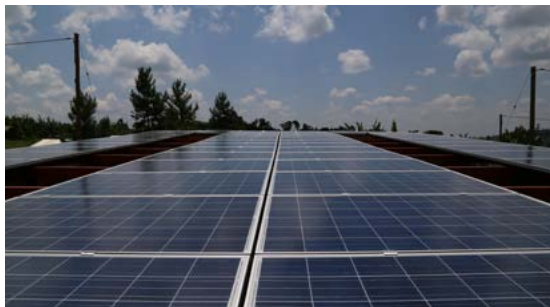
Top view of the Kanyegaramire mini-grid
