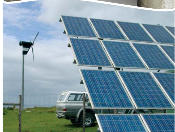
Battery charger - ECOTÈCNIA PV wind hybrid system South Africa - SMA
