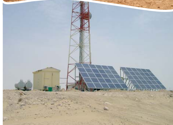
SHP power plant, Rwanda - MHYLAB Solar water pumping – PHOTOWATT PV system for telecommunication - SMA
